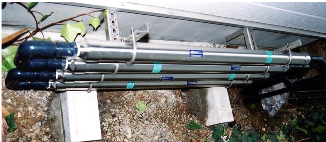
Installed at water source in parallel - TS - 1100 x 4
