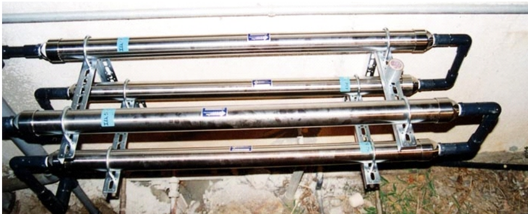
Parallel installation at the water source TS - 1100x 4
