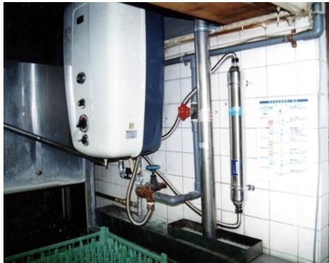
Installed at hot water source TS - 500 x1
