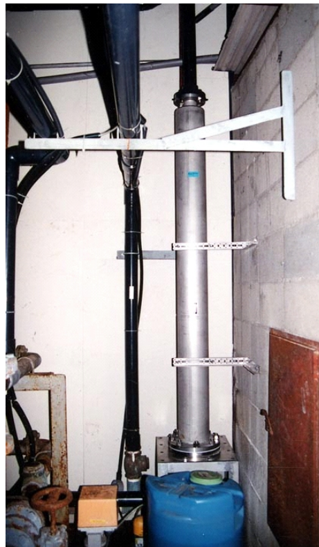
Installed at water source ST 150L x 1
